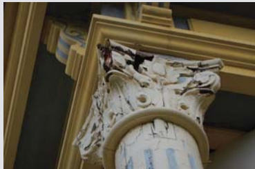
柱頭の腐朽 (本館車寄せ)
