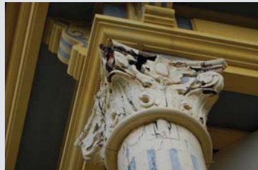
柱頭の腐朽 (本館車寄せ)
